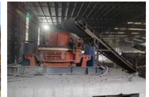
Hunan Limestone Project, Capacity: 500 tons per hour
