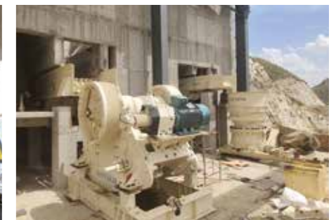
Gansu Lead-Zinc Ore Project, Capacity: 700 tons per hour
