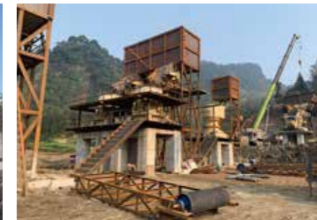
Yunnan Basalt EPC Project, Capacity: 400 tons per hour
